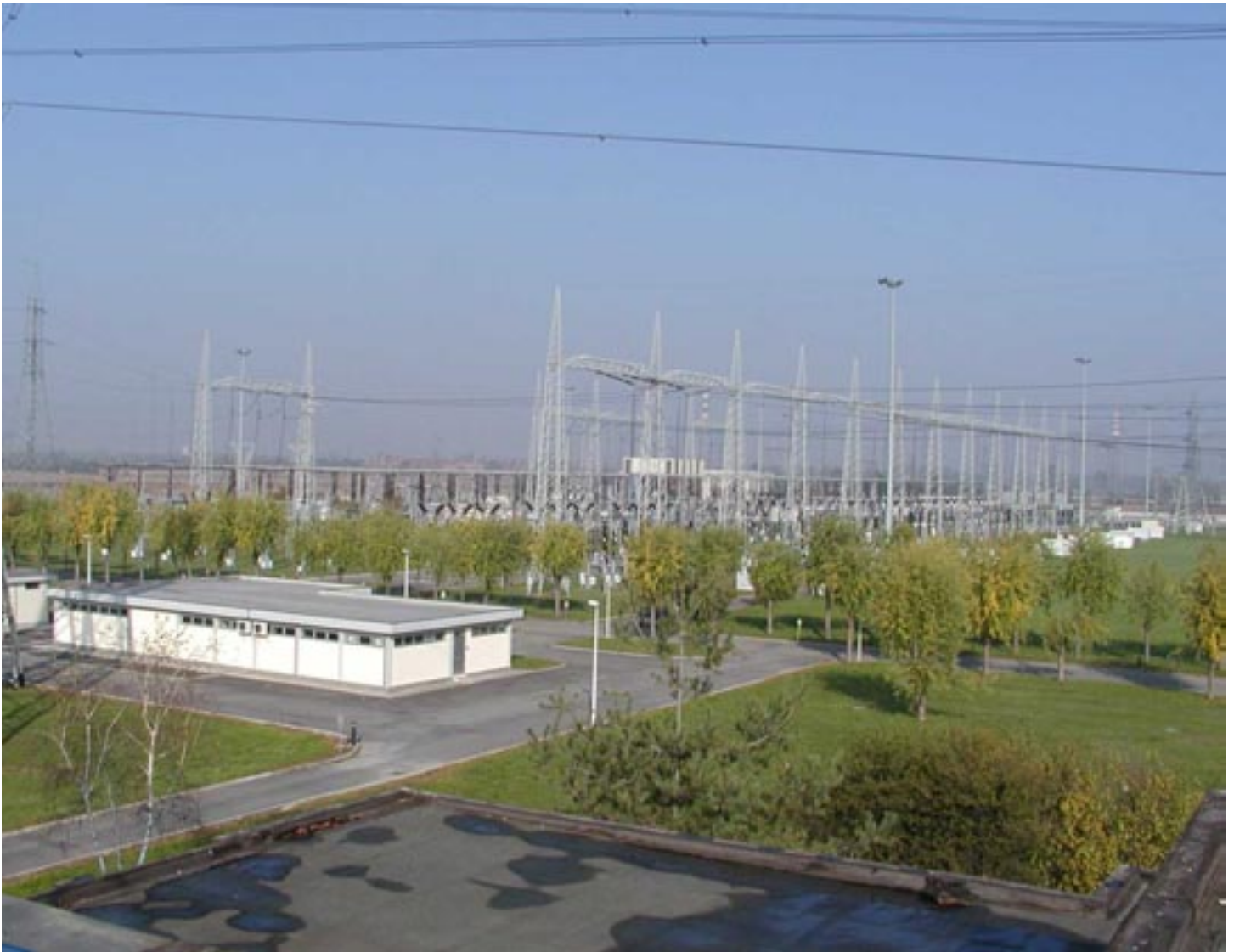
ENEL Center of Rondissone (courtesy of ENEL)
